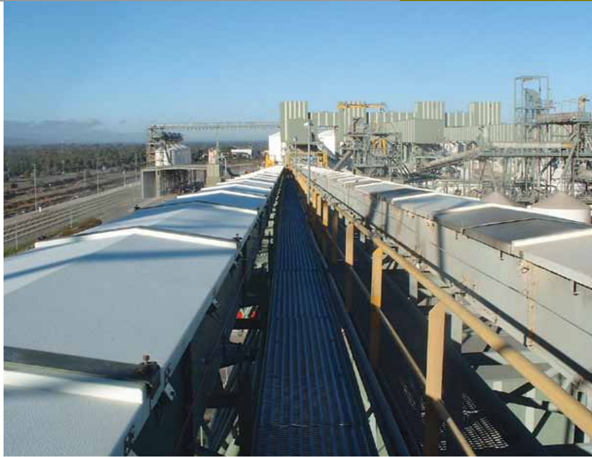
Joe White Maltings facility in Perth, with Aerobelt's conveyors shown before and after covers were fitted.
